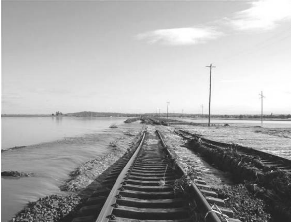
Damaged trackwork at Singleton (photograph courtesy of Michael Smith)
