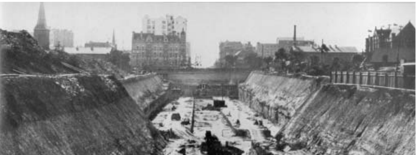
St James, with its innards exposed during construction of the City Railway. Two island platforms were built, the outer edges of each being used for City Circle traffic, the inner edges, destined for use on an Eastern Suburbs Railway were never used. The 25 trains per hour (one source says 26) arrived at the left-hand platform and travelled into tunnels under Macquarie St, to reverse and emerge on the right hand platform.
