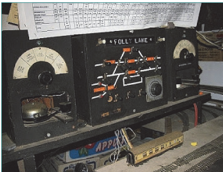
The Block Instrument (and loco. control rheostat) at Folly Lake, a station not present in the 1981 WTT. It replaced Sunbeam Colliery at some unspecified date.
